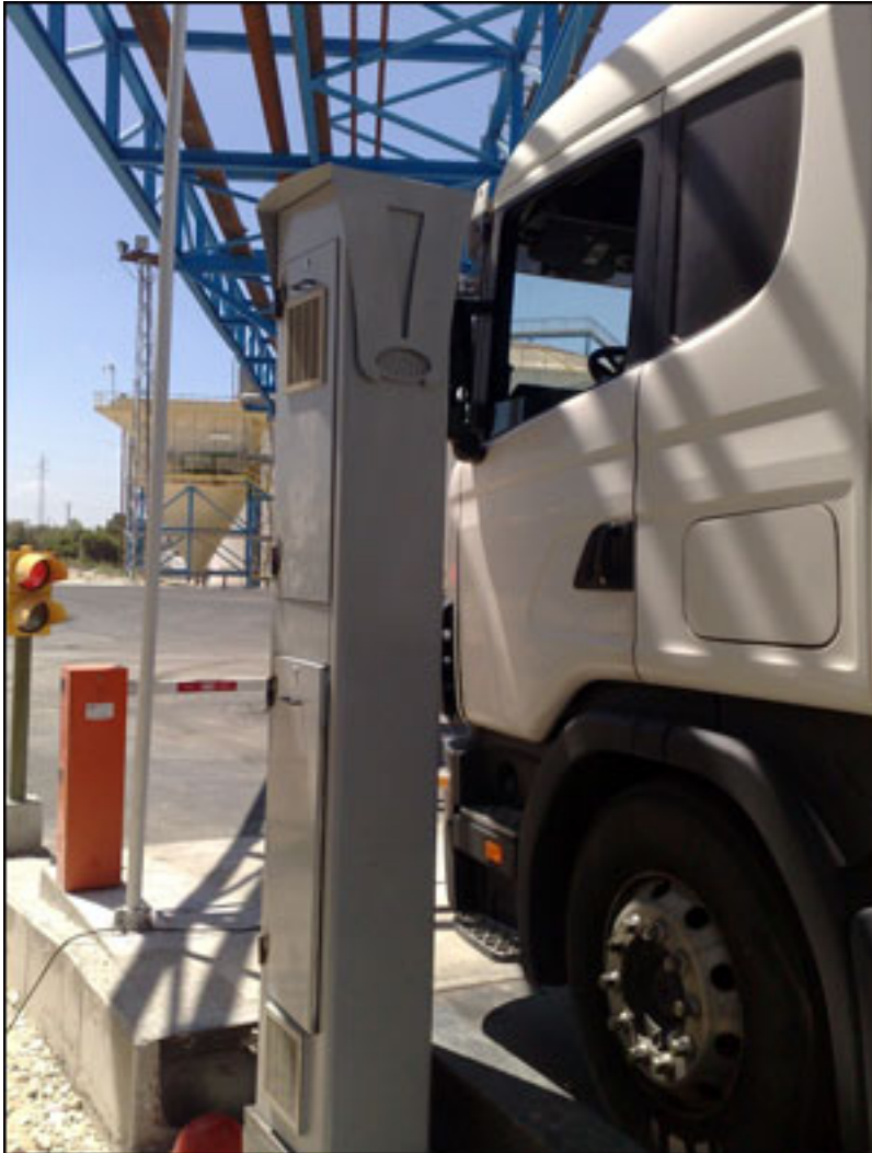
Identec Solutions' i-Port RFID readers are mounted at the refinery's entrance gates.
